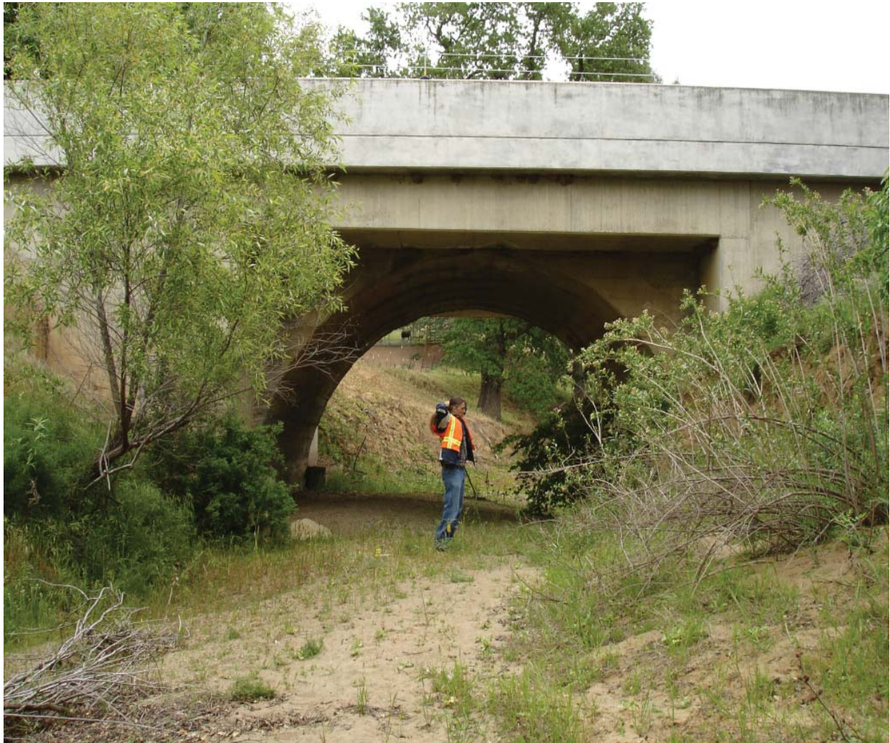
Figure 2. State highway bridge over stream channel. This under-sized bridge (relative to flows) provides only dry-season passage along riparian areas within an agricultural landscape.
